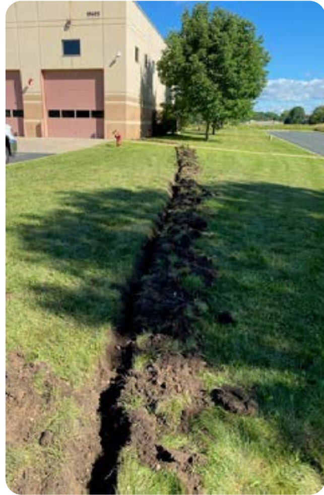
Staff dug a trench by hand to accommodate the cable for the new camera at Fire Station 2.
